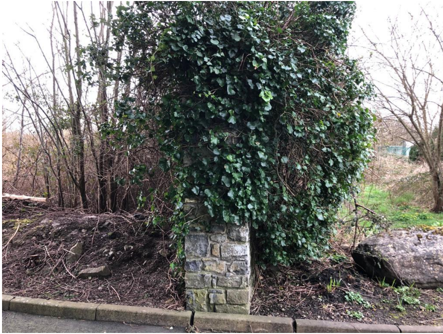
Pic 3: View south of the Boundary Wall which divides our site on the left from the adjacent existing 'Open Space' on the right.
