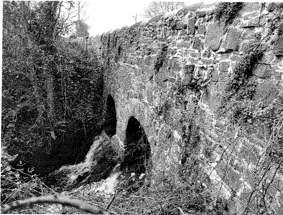
Plate 3 Ballynacally Bridge twin Arches and sudden drop in riverbed founded on bedrock adjacent to the Daly Bar Premises.
